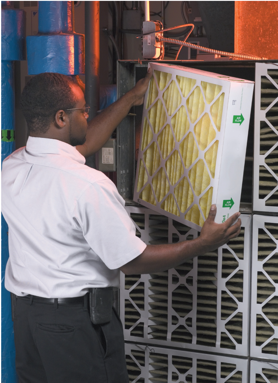
« Preventing bypass air is crucial when installing new filters.
